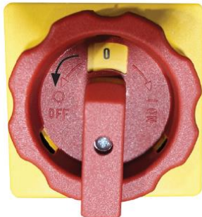
Figure 10: Main switch OFF
